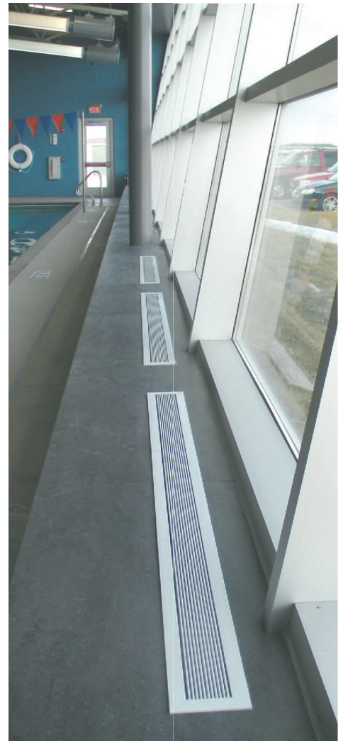
The BlueDuct® underground air duct supplies air to the linear diffusers in the natatorium area
