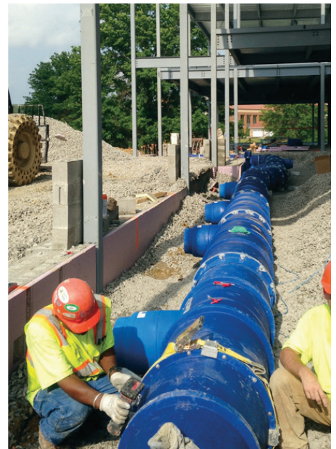
Installation of the The BlueDuct preinsulated Duct System at the Roberta A. Smith Library
